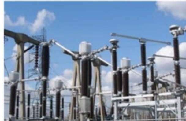
Typical 132kV AIS bay
