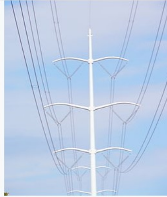
A double-circuit line
