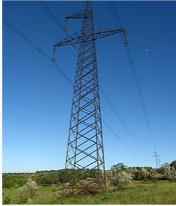
A single-circuit 330 kV line
