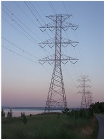
Four circuits on one tower line
